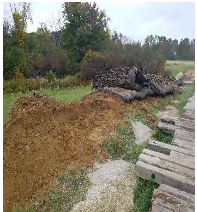
Fig 24: Maine Drilling and Blasting blasted bedrock at the Frink farm. Viewing east. (10-02-19).
