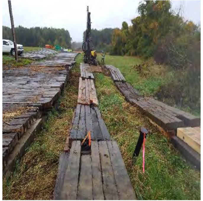
Fig 14: Maine Drilling and Blasting drilling exploratory borings at the Frink farm. Viewing west. (10-01-19).
