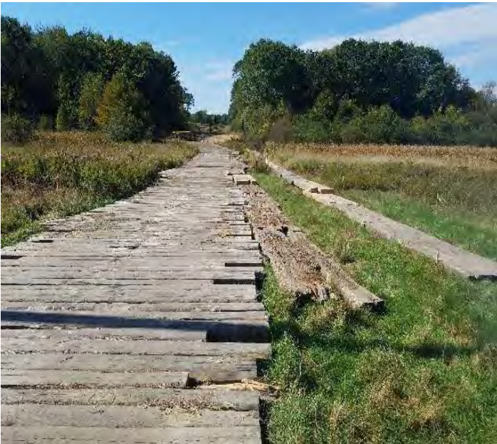
Fig 1: Placing timber matting on Frink farm, prepping for trenching activities. Viewing west. (9-26-19).
